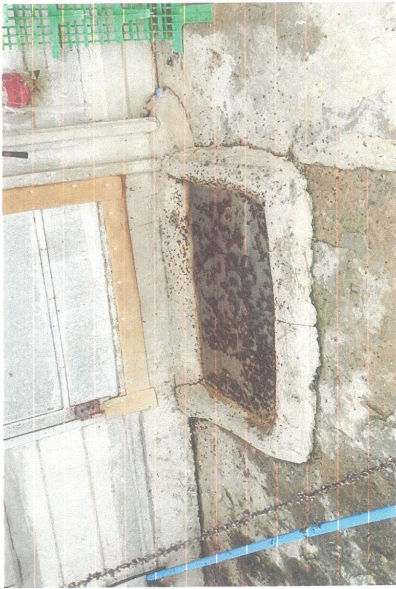
The flies dipped at the fly control solution at the vicinity of the tunnel vent.
